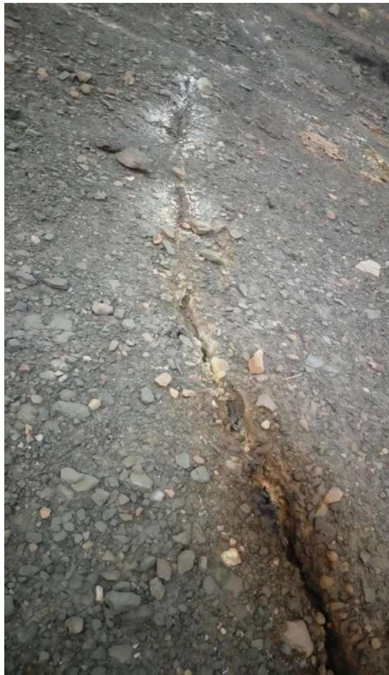
Figure 20: Fume cracks in the Bhulanbarari area.
